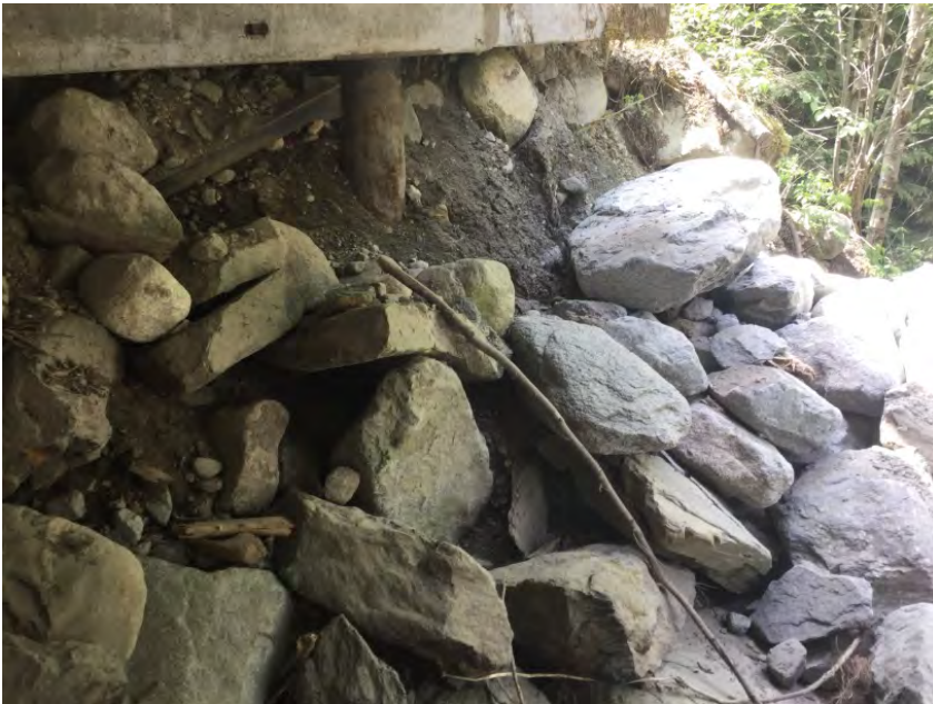
Downstream left pipe column partially exposed with little riprap in front
