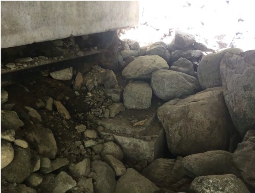
Upstream right bank pipe column and footing partially exposed
