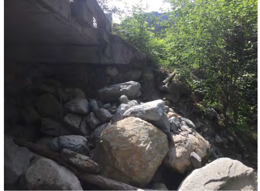
Downstream left bank fill erosion
