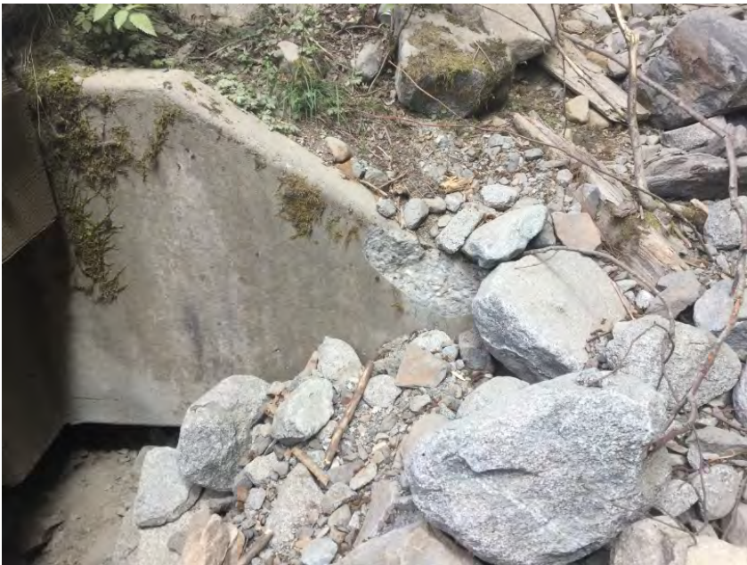
Minor damage noted to upstream right bank ballast wall
