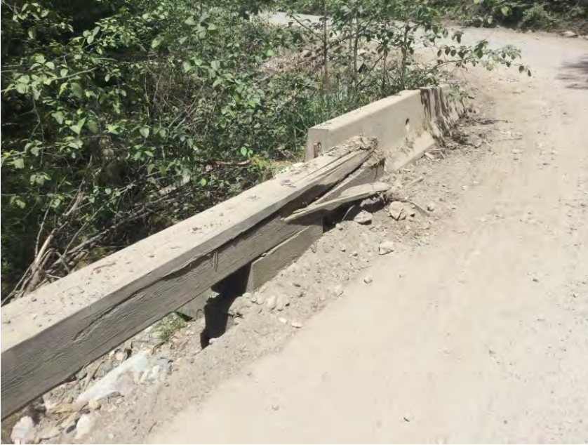
Damaged guardrail downstream right bank
